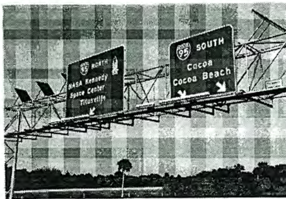
Figure 10a-8. PV-powered guide sign lighting system.
