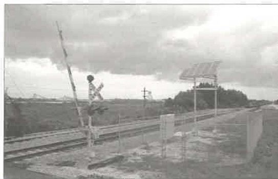
PV-powered railroad crossing – Cocoa, Florida (June 1982)
