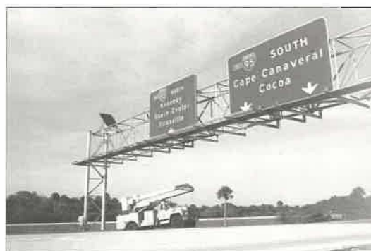
PV signs on Beeline Highway
