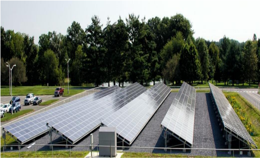
NIST Ground mounted PV array located in Gaithersburg, MD.
