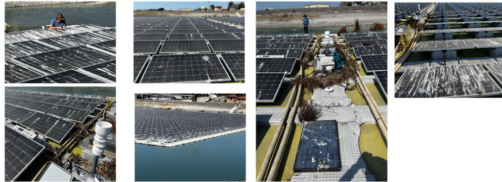
Bird droppings, after three years in operation, on a 1.7 MW Floating solar PV at a water treatment facility, Windsor, CA
