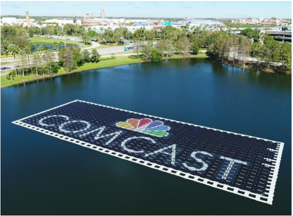
Universal Studios Orlando Builds Floating Solar Array
