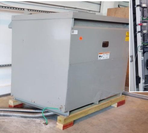
Step up Transformer: 500 KVA (480 V/600V)
