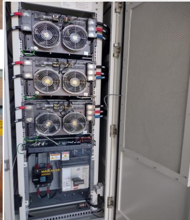
Power Conversion System (PCS) 500 KVA
