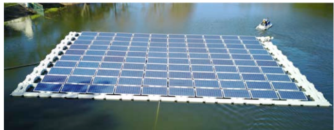
FSEC is leading a nationwide research project on floating solar systems like this one located in Orlando. Photo: Orlando Utilities Commission
