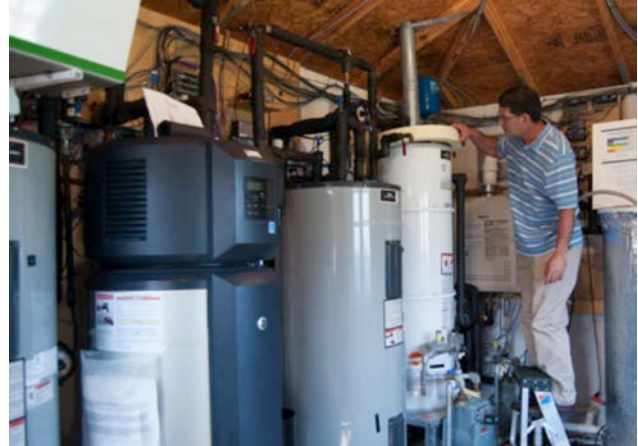
FSEC's Hot Water Systems Lab is used to evaluate a variety of hot water systems simultaneously and side-by-side to compare energy performance and time of day electric loads.
