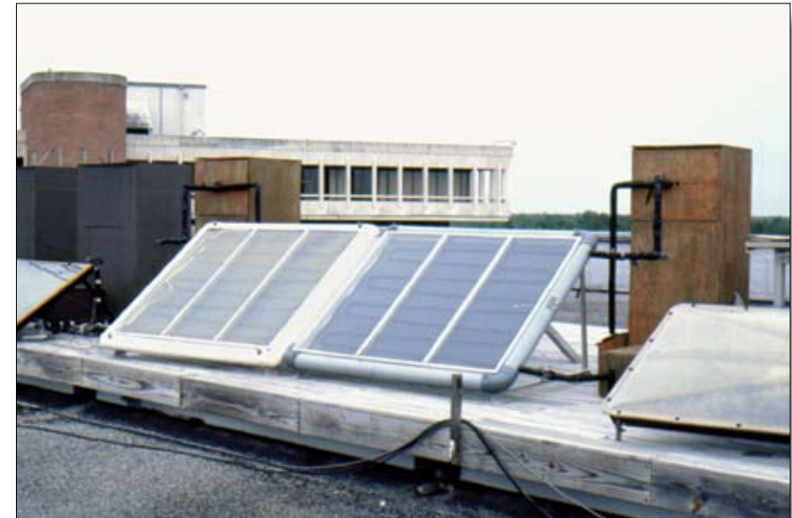
Solar hot water system demonstration project on roof of UCF Engineering Building in 1974-75. This UCF project was under the direction of Dr. Bruce Nimmo, who later became an FSEC employee and Director of the Advanced Technologies Division.
