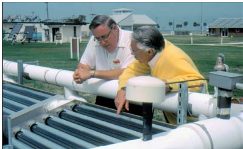
Solar air conditioning project R&D Building - Omar Hancock (left) explaining to a visitor (February 1979)
