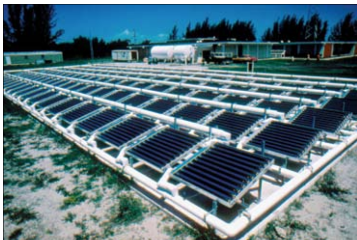
GE evacuated tube collector field for FSEC solar air conditioning project (1979)
