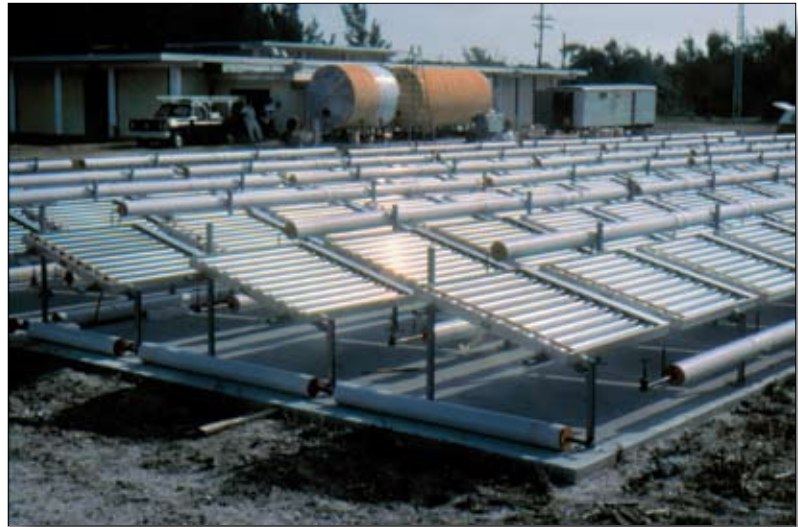
Solar air conditioning project R&D Building - evacuated tube collectors (February 1979)
