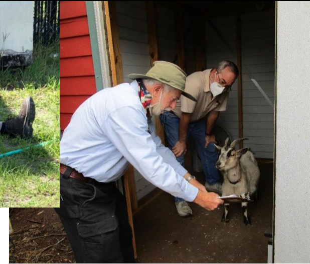
Bill Young and David Bittle explaining the PV repairs to one of the schoolyard residents living near the array.
