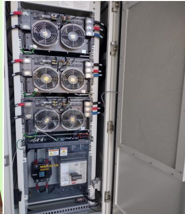
Power Conversion System (PCS) 500 KVA
