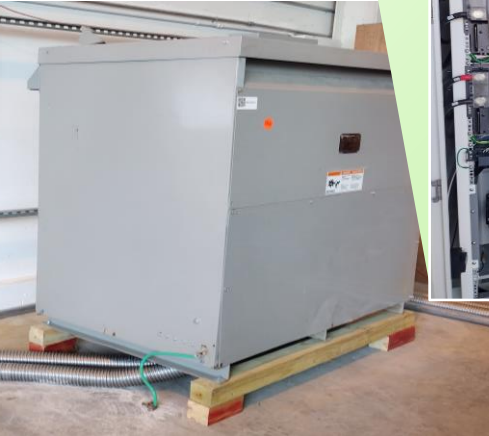
Step up Transformer: 500 KVA (480 V/600V)
