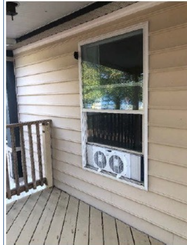
c. Window fan installed in the MZ providing outdoor air into the home. This strategy pressurizes the main zone, resulting in a lesser pressure in the closed-off IZ w.r.t. MZ, which helps with containment.
